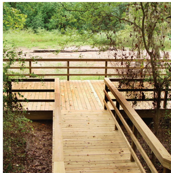
One of our newly constructed viewing decks at swamp level on the blue trail
