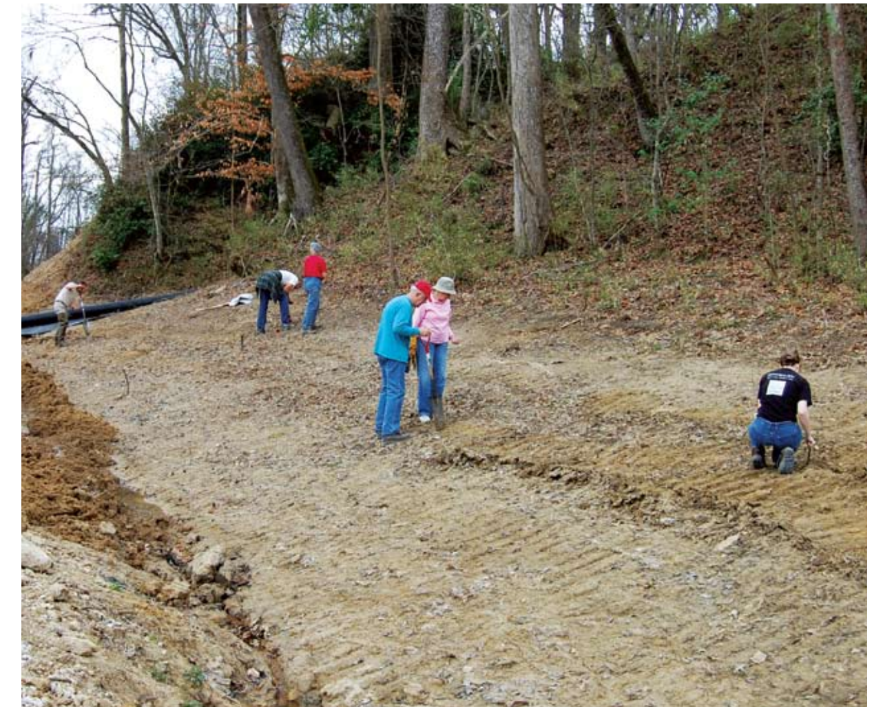
Museum Staff and Volunteers plant a variety of trees and acorns along the bluff at the water pipeline work site.
